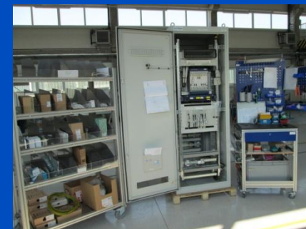
Cubicle workstation with worktable & holder cart
